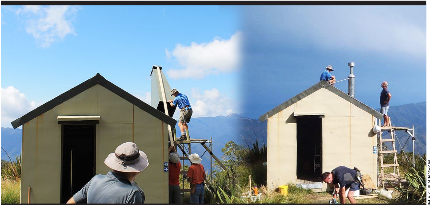
Out with the old; in with the new. The original iron chimney was toppled, and replaced with a modern one.
